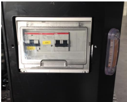
15. Main differential panel
