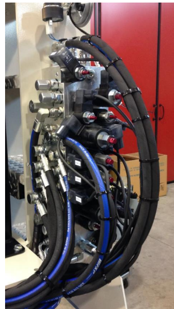
14. Main hydraulic unit
