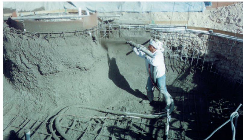
The LS500, with its powerful ability to handle the toughest shotcrete mixes, enables a swimming pool contractor to apply shotcrete to two pools a day.
