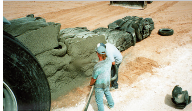
Shotcreting (wet gunning) with a stiff, low slump mix, is just one of the many uses for the LS600 concrete pump.
