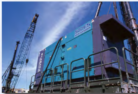
As the power source in the construction site.
